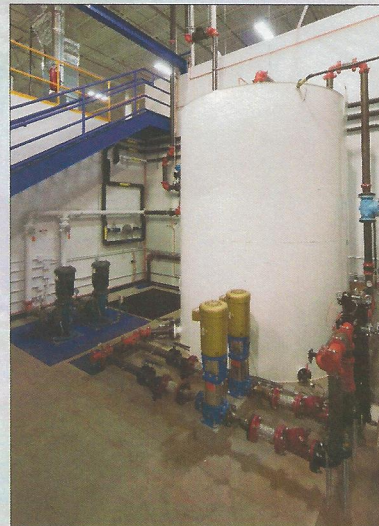
A 4,000-gallon water supply tank provides ample process water to maintain engine temperatures throughout test sequences.
